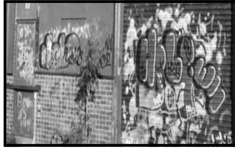
Graffiti found by local councillor's in West Shoebury which has been reported to the Council
