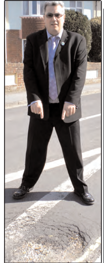
Road in the hole: Geoff says he will tackle Hampshire Highways to repair this pot hole in Jubilee Road – one of many left by the big freeze.
