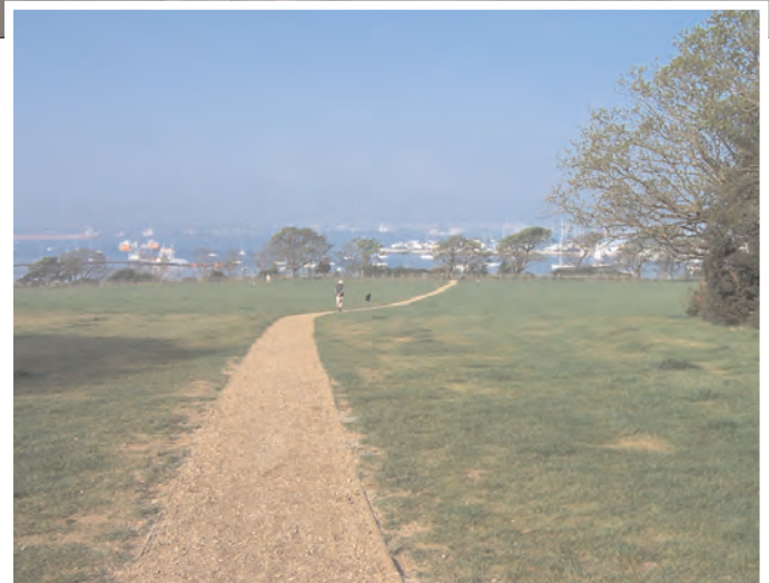
Pathways to success: Work proceeds apace to resurface pavements in Warsash Road (top), while the Strawberry Field path has been reinstated (above).
