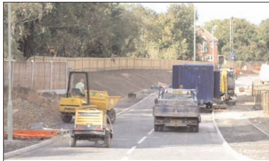
Almost there: Picture taken earlier this month shows finishing touches being put to the new link.
