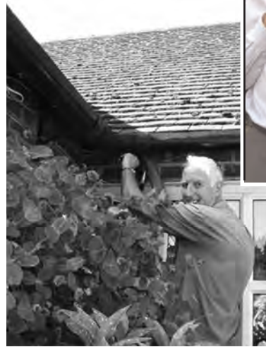
Up a ladder: David rolls up his sleeves to help repair the roof at Sarisbury Parish Rooms.
