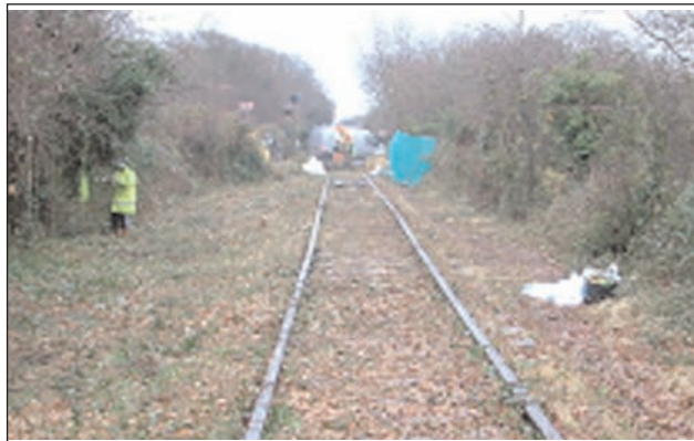
Flashback: Preliminary work to clear the overgrown rail track started at the beginning of the year.
